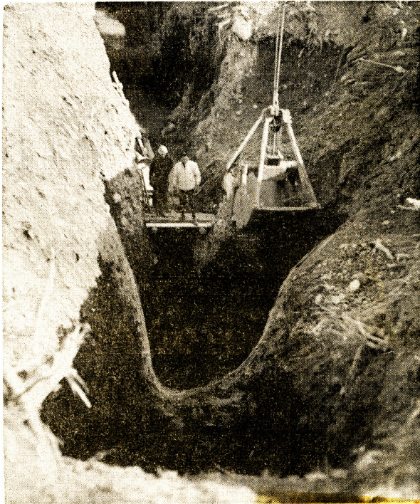
Dwarfed at Oak Island's newly-found shaft are two men and a large digging bucket. Robert Dunfield believes the new find is part used to flood the treasure site. (Brigley Photo)
