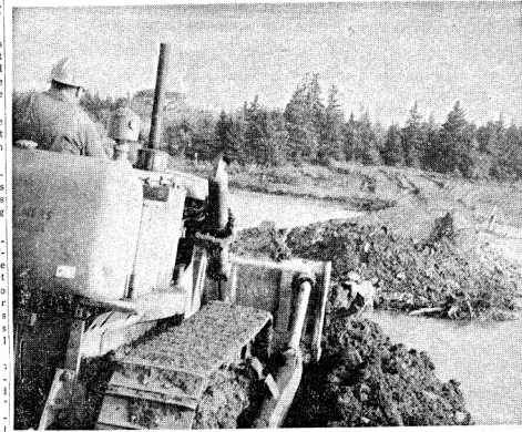
Bulldozer fills in the last gap of the temporary causeway at Oak Island. (Brigley photo)
